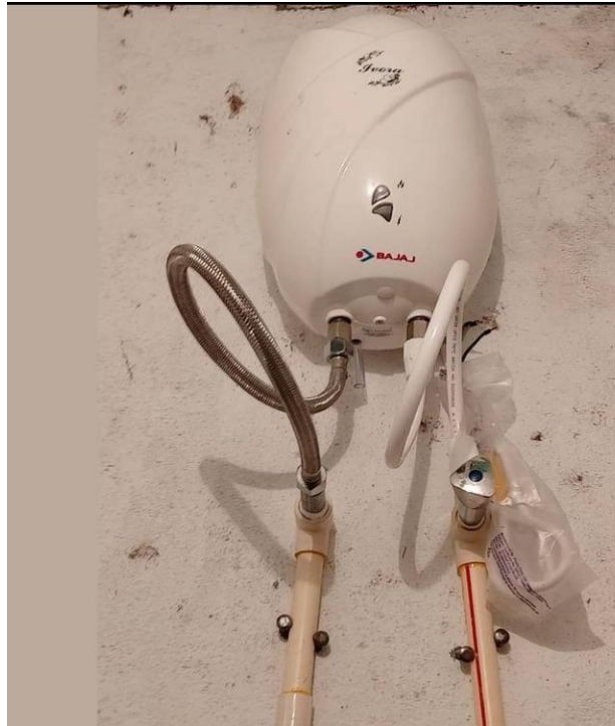
Picture of Geyser Installation at Old Age Home
