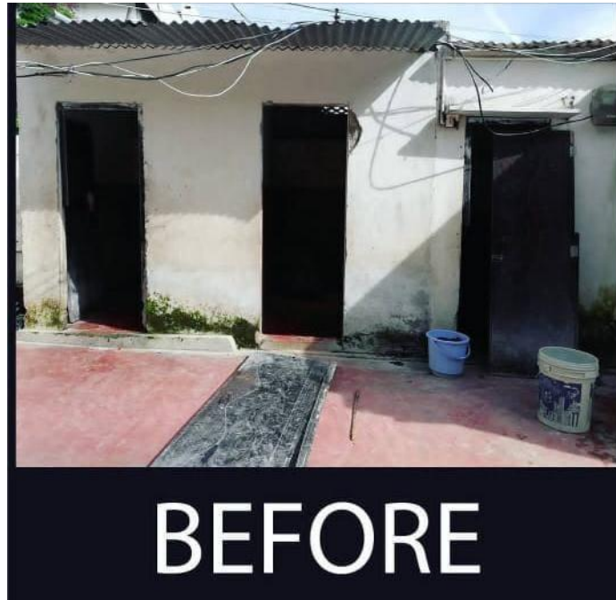
Image showing restrooms without doors
